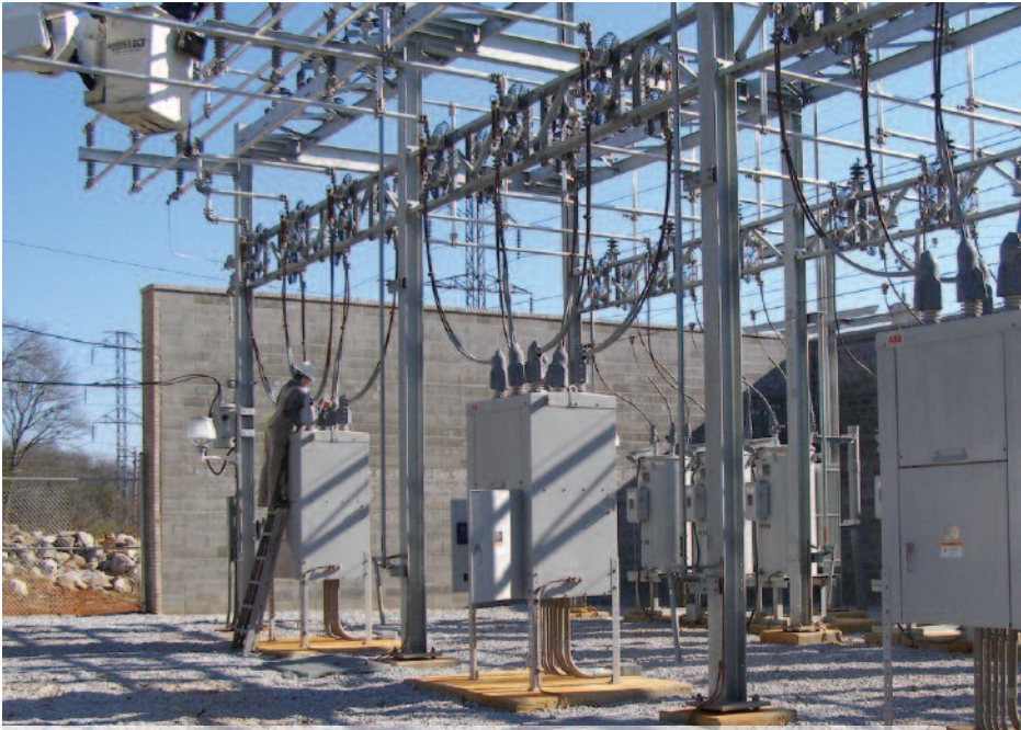
A Huntsville Utilities electrician works on connections in the new Garth Mountain Substation serving the growing Jones Valley portion of Huntsville.
